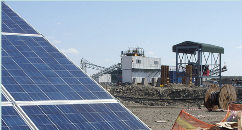
Figure 4: PV installation at Thabazimbi Mine
